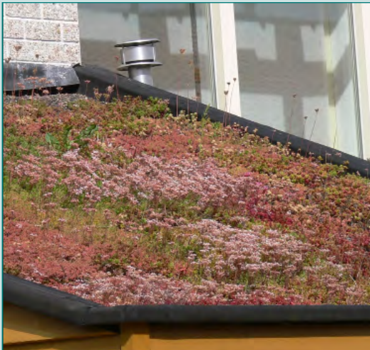
AN EXTENSIVE GREEN ROOF SHOWING A RANGE OF SEDUM COLOURS PHOTO: LAMIOT (WIKIMEDIA COMMONS)
