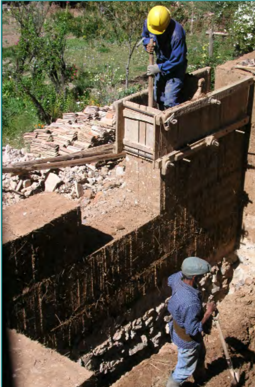
RAMMED EARTH WALLS AND FLOORS UNDER CONSTRUCTION IN PERU: JYB DEVOT, CC BY-SA 4.0, VIA WIKIMEDIA COMMONS
