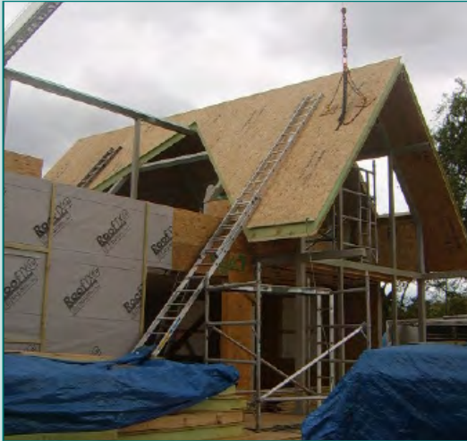
SIPS PANELS BEING ERRECTED IN A DOMESTIC SITUATION PHOTOS COURTESY SIPS UK LTD.
