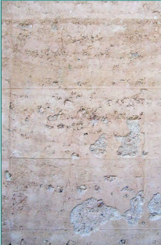
CLOSE UP OF A RAMMED EARTH WALL PHOTO: ANDREW DUNN (WIKIMEDIA COMMONS)
