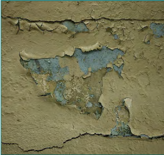
PEELING PAINT PHOTO: PHOTO: DANIEL SCHWEN (WIKIMEDIS COMMONS)
