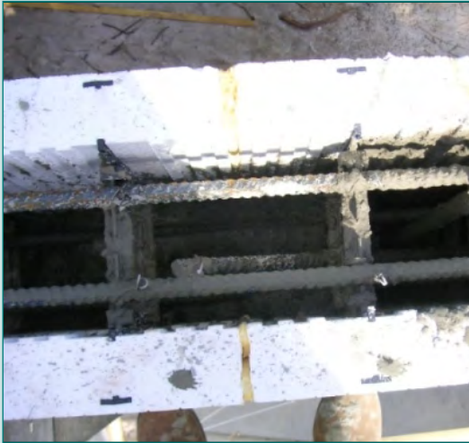
A CLOSE-UP TOP VIEW OF ICF BLOCKS UNDER CONSTRUCTION PHOTO: MIKEOG39 - HTTP://WWW.WISEHOMEDESIGN.COM
