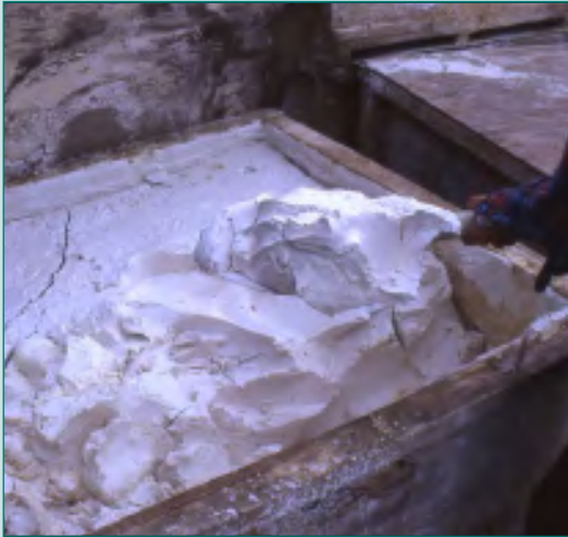
LIME SETTLING TANK PHOTO: JJ SHARPE
