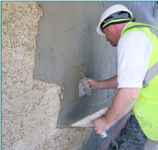
LIME RENDER BEING APPLIED OVER HEMCRETE BASE PHOTO: COPYRIGHT © 2000-2009 LIME TECHNOLOGY LIMITED
