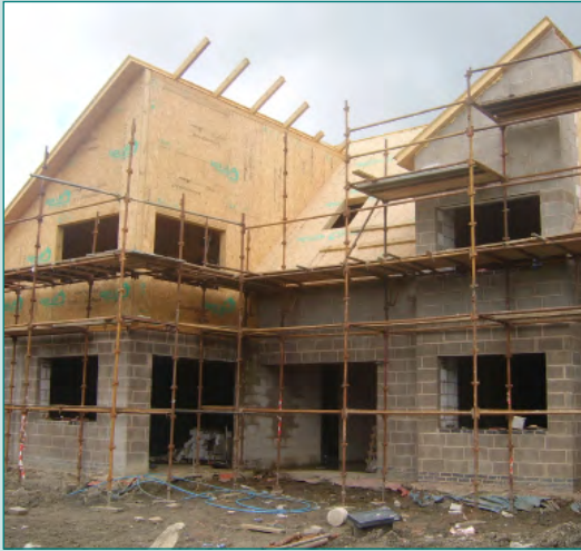
SIPS PANELS BEING ERECTED IN A DOMESTIC SITUATION PHOTOS COURTESY SIPS UK LTD.
